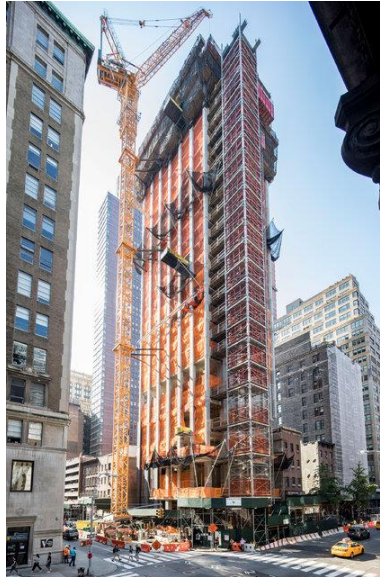
Construction on 277 Fifth Avenue, in the NoMad neighborhood of Manhattan. Credit Katherine Marks for The New York Times
